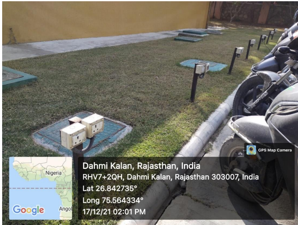
Picture 8: EV charging points .
